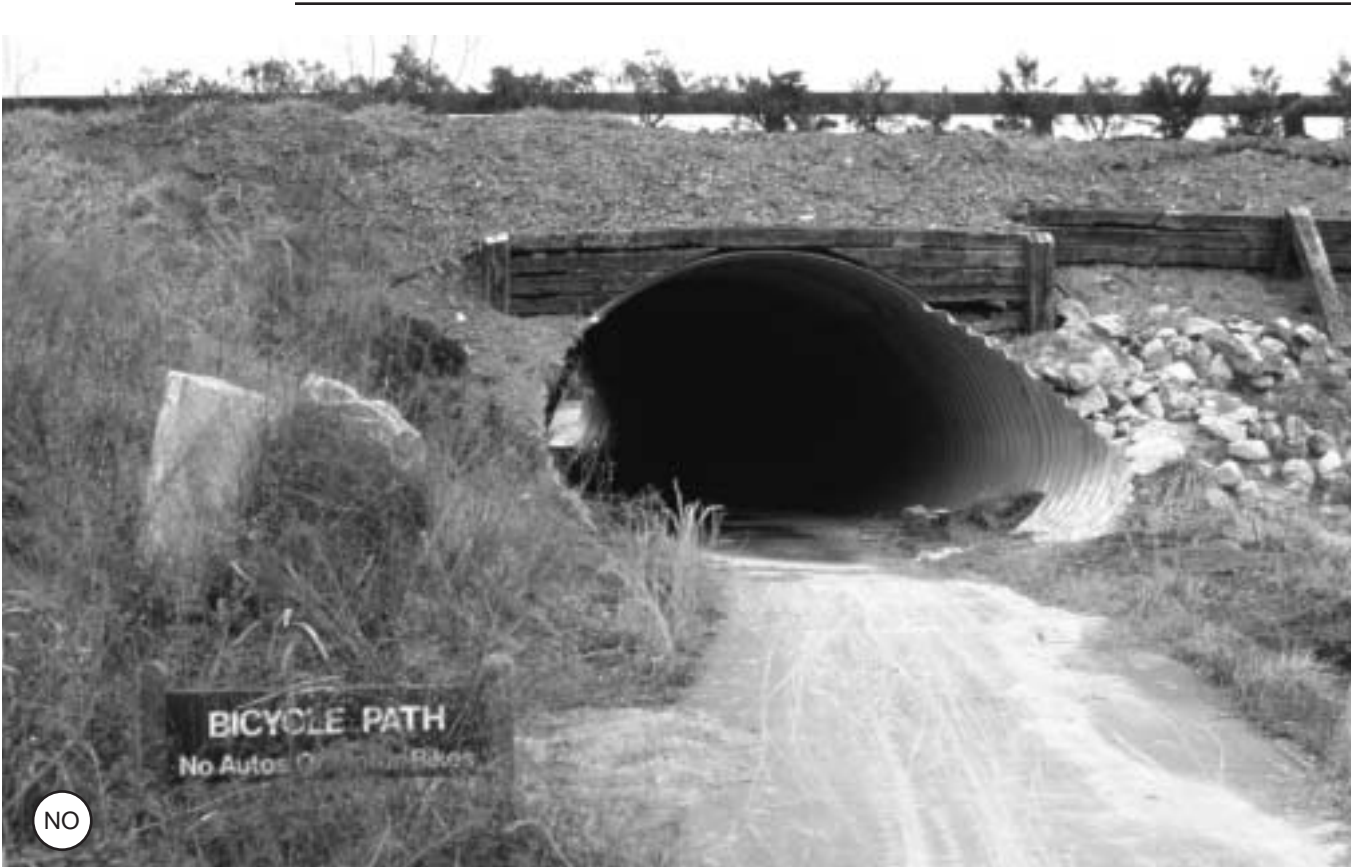
Figure 4-50: Path lighting is particularly important where ambient light levels change dramatically, as in an underpass.
